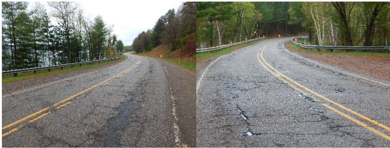
(a) low temperature cracking and fatigue cracking
